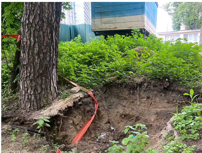
Fig. 2.2. Landslide near the construction of a metro tunnel
