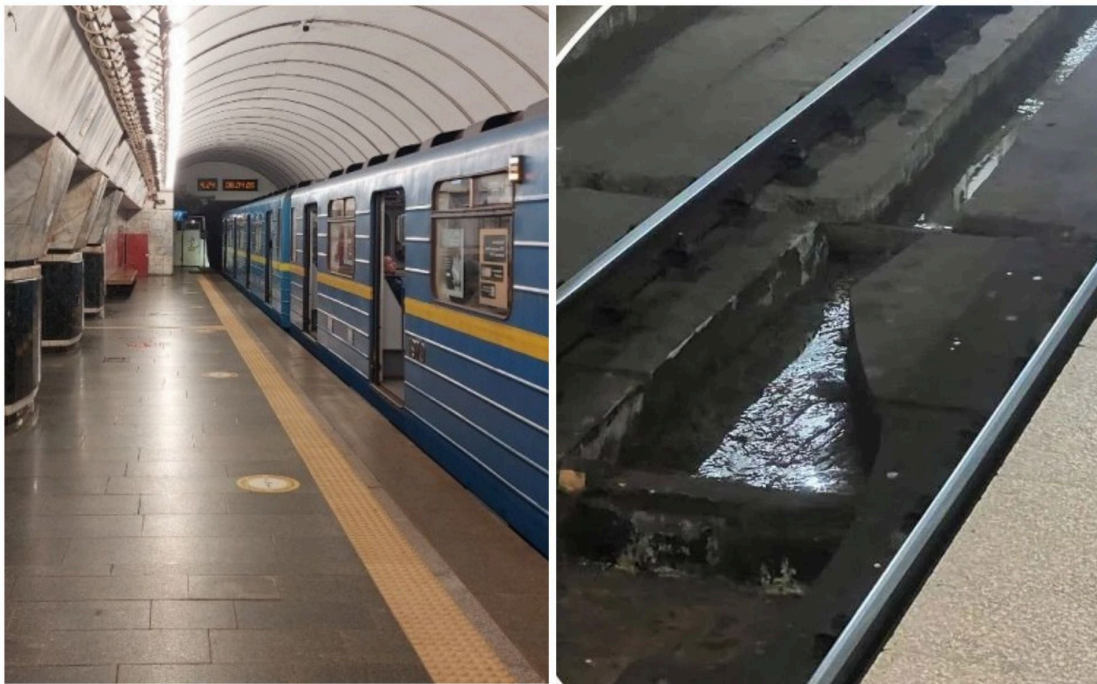
Fig. 2.3 groundwater infiltration into the metro tunnel
